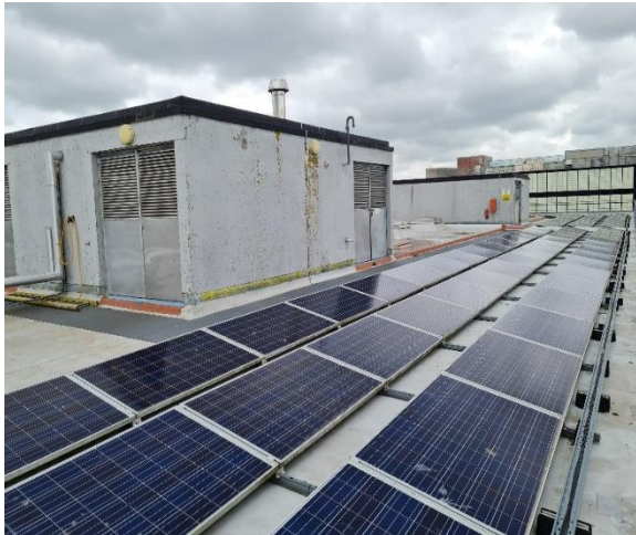
Figure 38: During a previous project the Business School already had 160 PV panels installed
