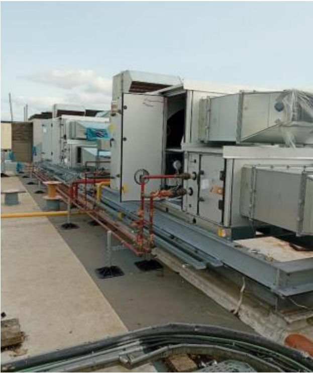
Photo 37: New AHU plant installed as part of the Deep Fabric Retrofit
