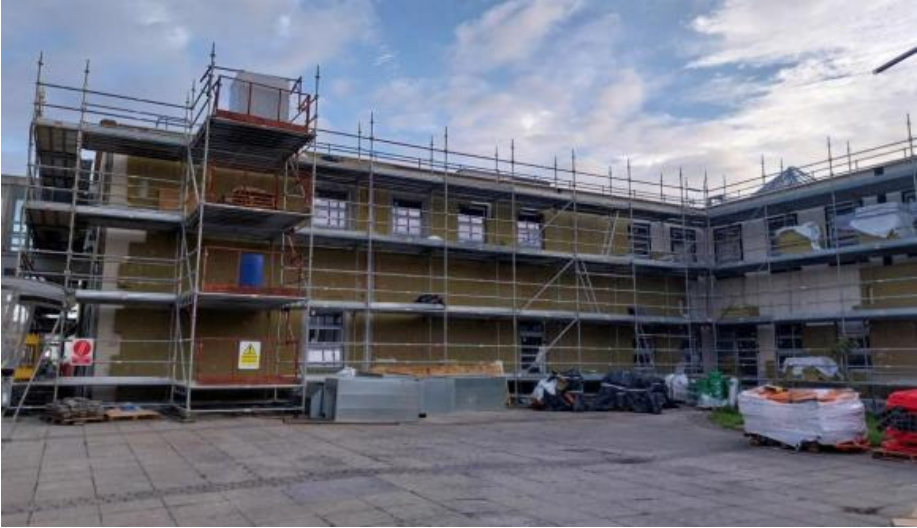
Figure 36: Deep Fabric Retrofit of Business School with installation of new external render in progress
