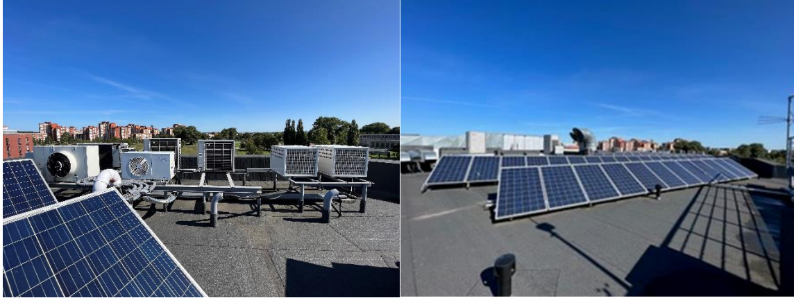
Figure 28. The roof of the MRI building with solar panels and BMS equipment
