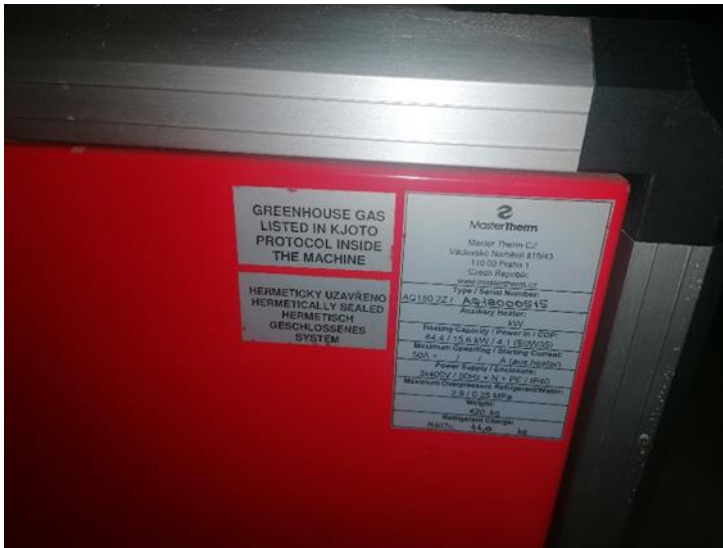
Figure 30. The greenhouse gas containment equipment
