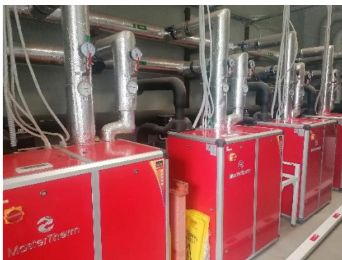
Figure 29. The geothermal power plant's equipment (heating pumps)
